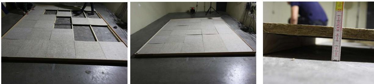
photo : Test n° 17 : details during placement of the rockwool panels on the wooden frame with a height of 45mm.
